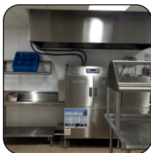
Ware washing area
